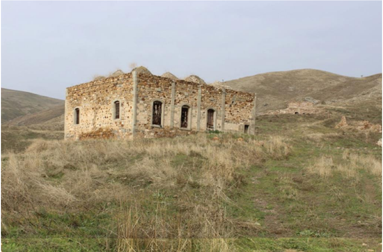
Images 18–21: Qochahmadli Village Mosque, Fuzuli (XVIII century. Vandalized and partially destroyed after the occupation of Fuzuli in 1993. Was used as a cattle shed)
